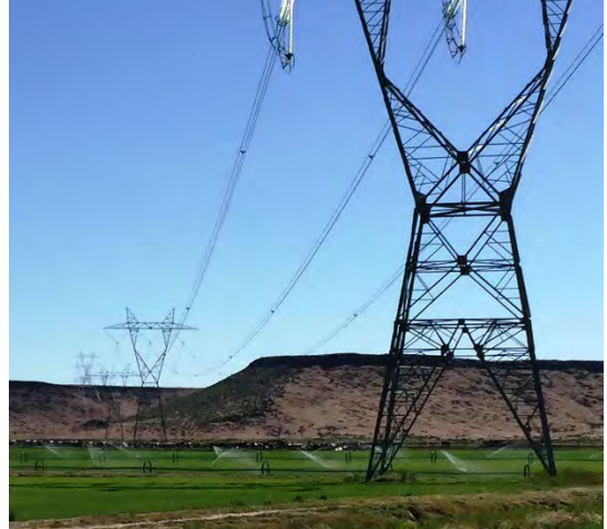
500-kilovolt (kV) transmission line near Melba, Idaho
