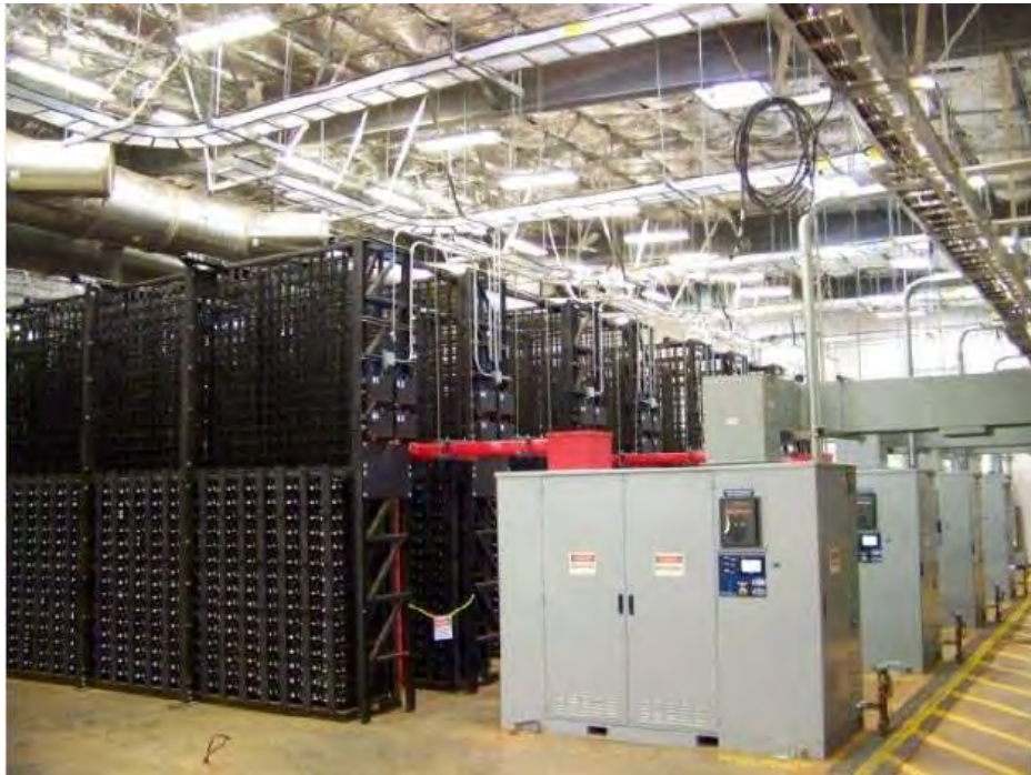
Figure 13 - PowerCell™ Stacks with PCS
