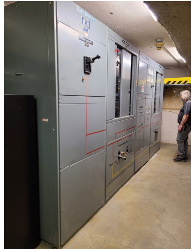
Existing 208/120V Main Switchboard located in basement
