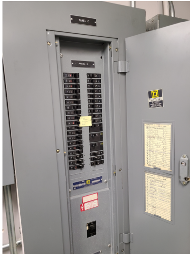
Existing age of Panelboards in Building
