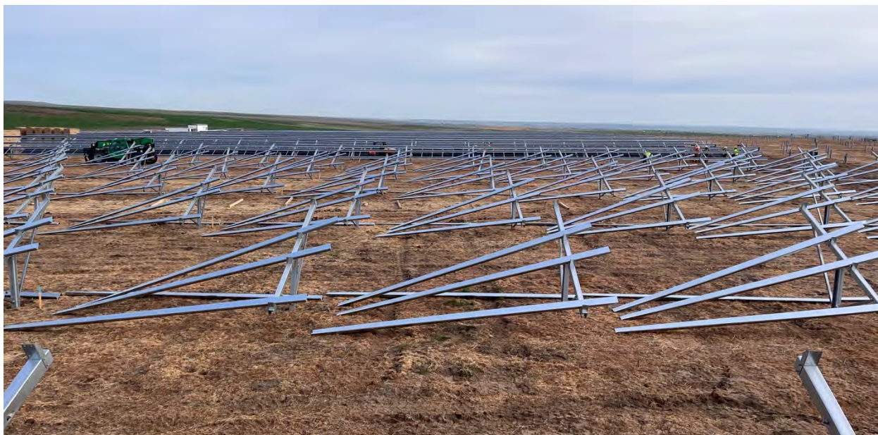
Photo 2. Racking, panels, inverters at Pilot Rock Solar 1 (taken April 11, 2024)
