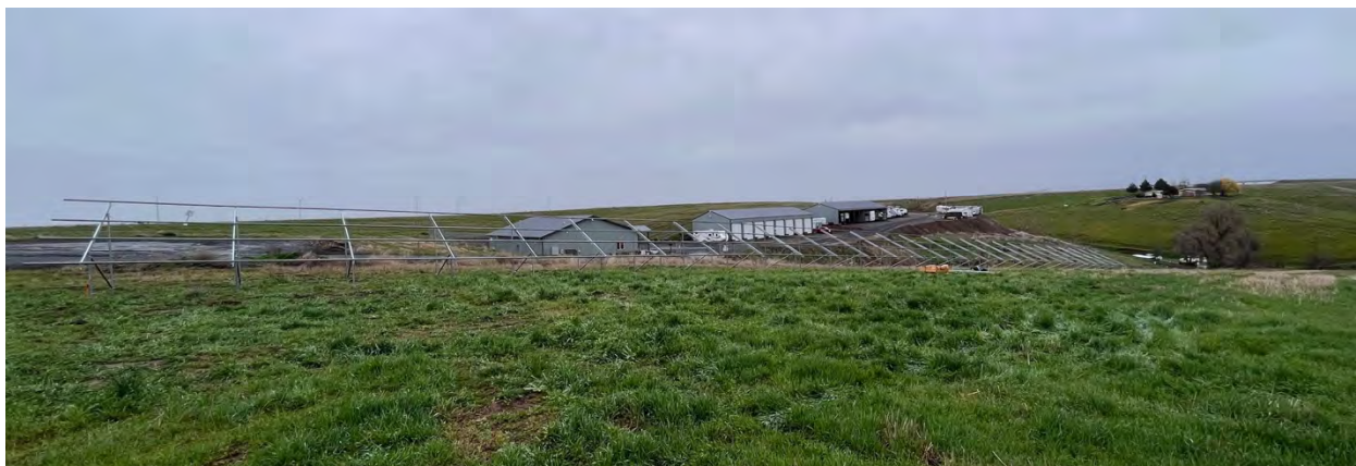
Photo 3. Row of racking installed at Buckaroo Solar 1 (taken April 11, 2024)
