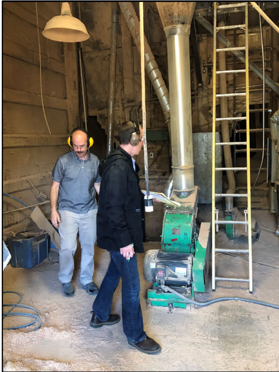
One of the 25 HP blowers used in the multi-building dust collection system.
