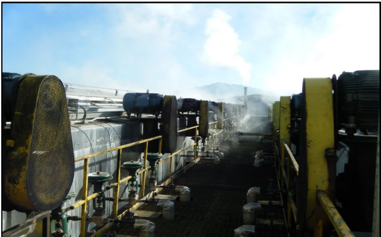
Kiln-12 - 20 HP fan motors and steam valves.
