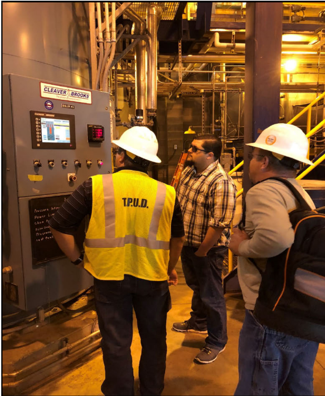
Cleaver Brooks 5 MW Electric Boiler - Derek Mickelson and Glenn Johnston on site with TCCA engineering staff to ensure the breaker relay would coordinate properly with the PUD switch gear that provides service to the boiler.
