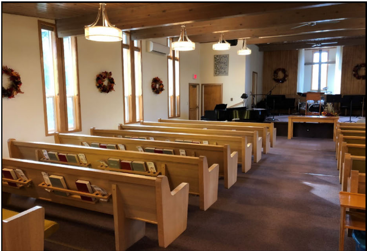
Ductless Heat Pump Unit #1 – Installed in the Sanctuary.
