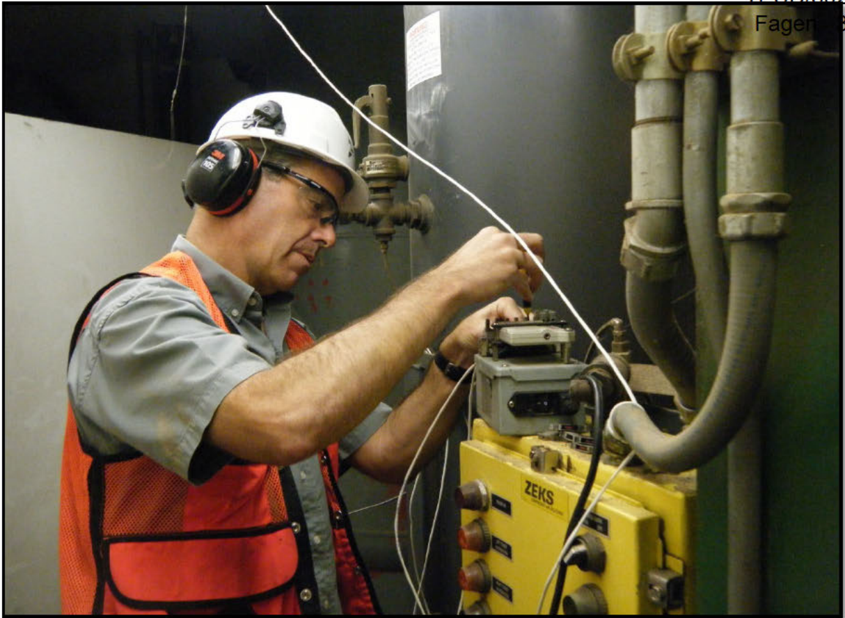
Tim Dugan with Compression Engineering – Installing a data logger to record energy use on the ZEKS air dryer.
