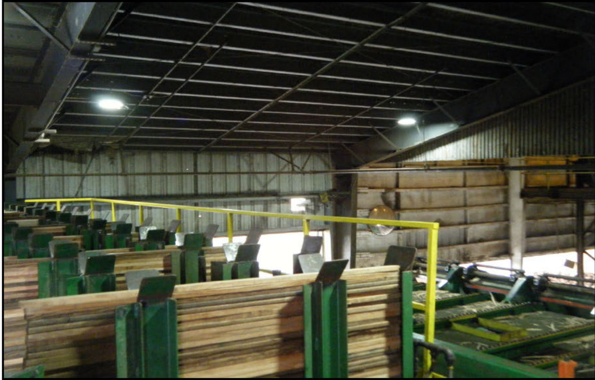
Saw Mill #2 Stacker – 150 watt LED fixtures installed.
