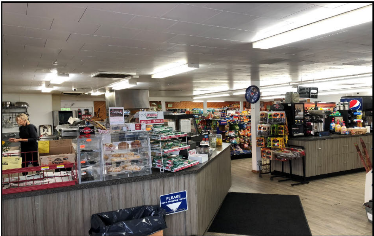
Interior Lighting – Retrofitted the 8 foot, 172 watt fluorescent fixtures, to 48w watt LED.
