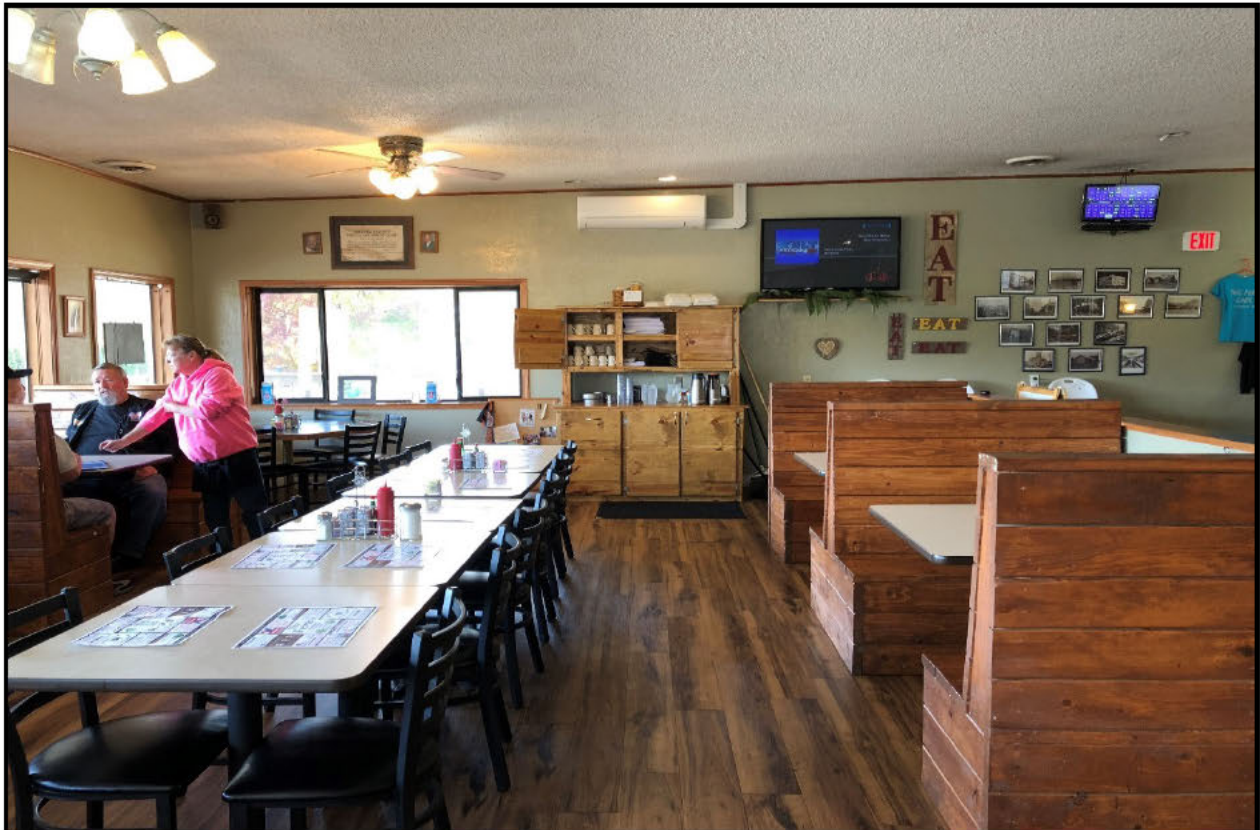
The Fern Restaurant – Ductless Heat Pumps Installed.
