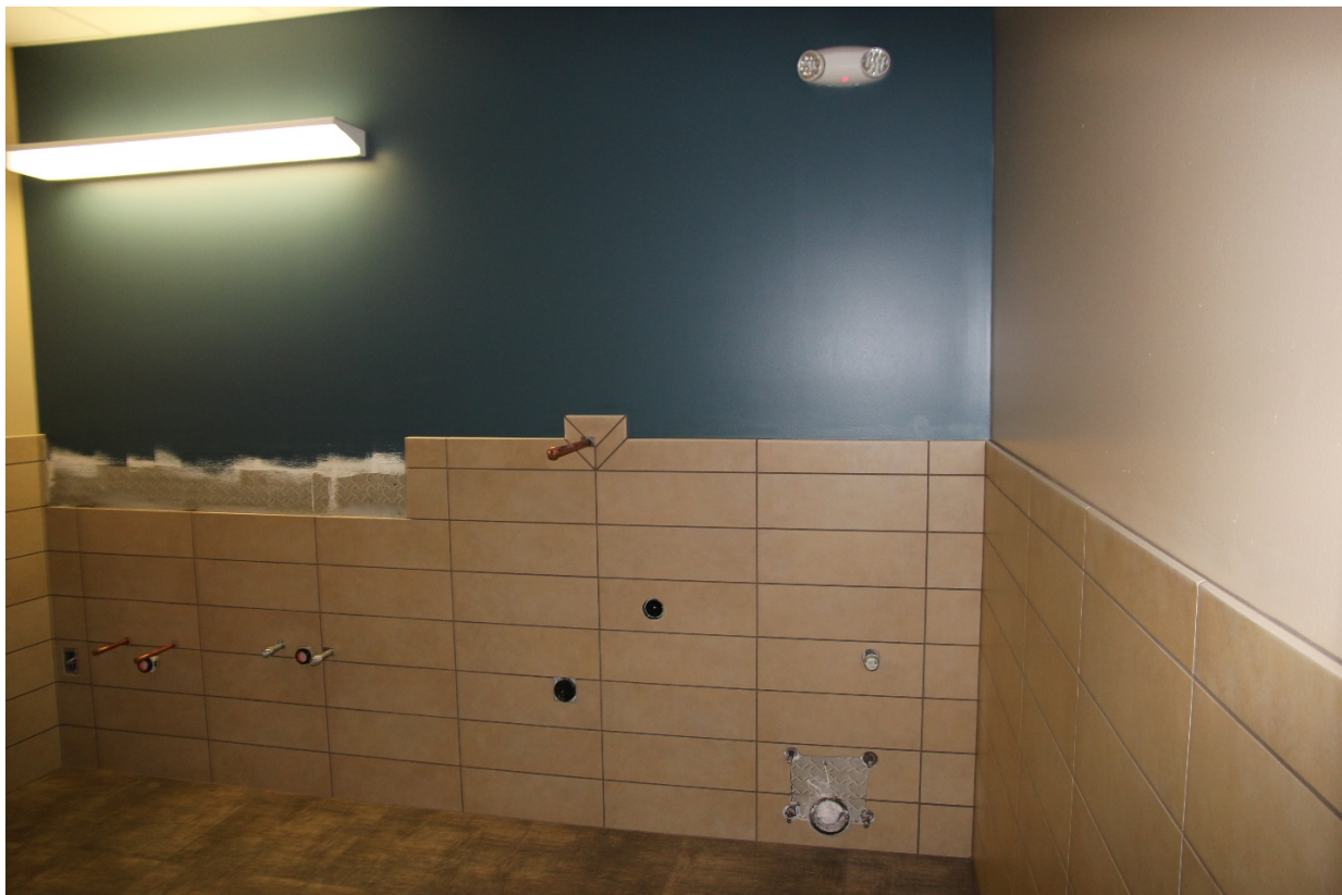
New restroom under construction. Touch less low flow fixtures were installed to conserve water.
