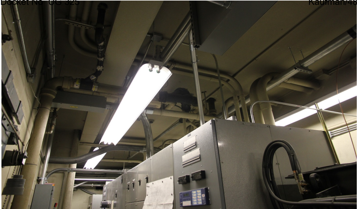
This photo shows new floor drain in top left corner just above the main switchgear. The drain protects switchgear from flooding in bathrooms directly above.
