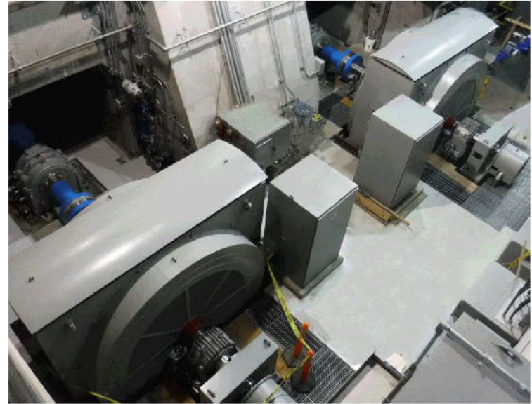
In 2016, the last two (of four) original turbine generating units at our 108-year-old Nine Mile Powerhouse were replaced with new, more efficient units as part of a multi-year project to increase the generation of clean, renewable, low-cost hydropower.
