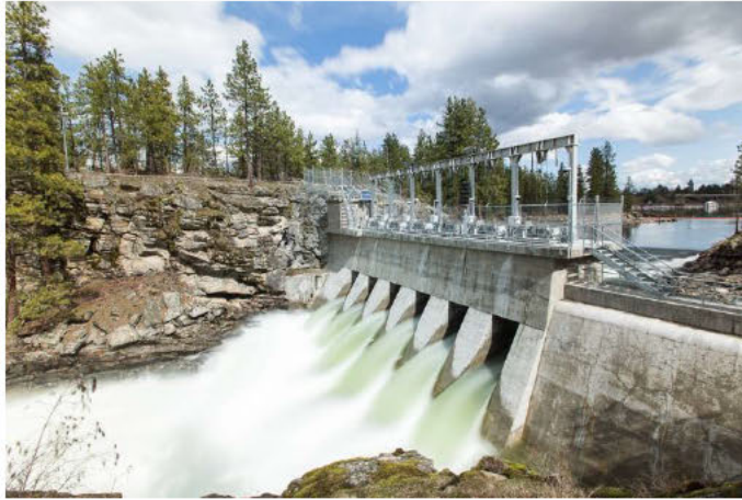
The 110-year old Post Falls South Channel Dam was officially returned to service after a two-year rehabilitation in February 2016.
