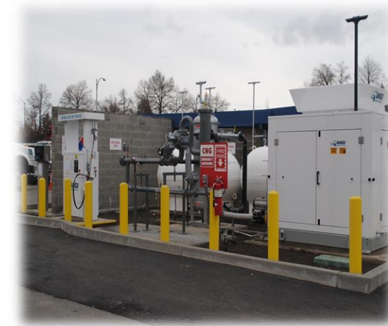
Mission Avenue Refueling Station - Spokane
