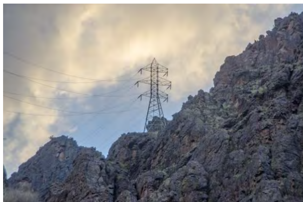
Idaho Power's double-circuit 230-kilovolt (kV) transmission line traversing Hells Canyon.
