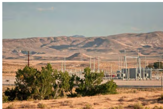
View of the Hemingway Substation.
