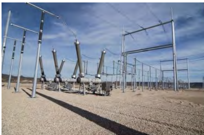
The Hemingway Substation in southern Idaho is a major hub for power running through Idaho Power’s transmission system.
