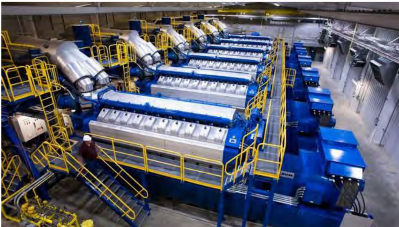
Engine Hall at Goodman Energy Center Kansas
