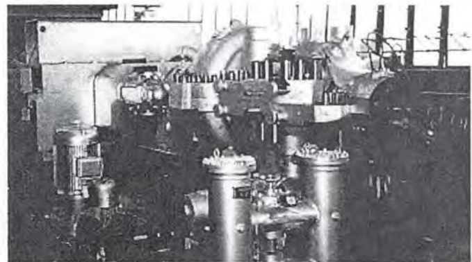
Ceske Budejovice, Czech Republic: 29 MW back-pressure turbine for district heating plant
