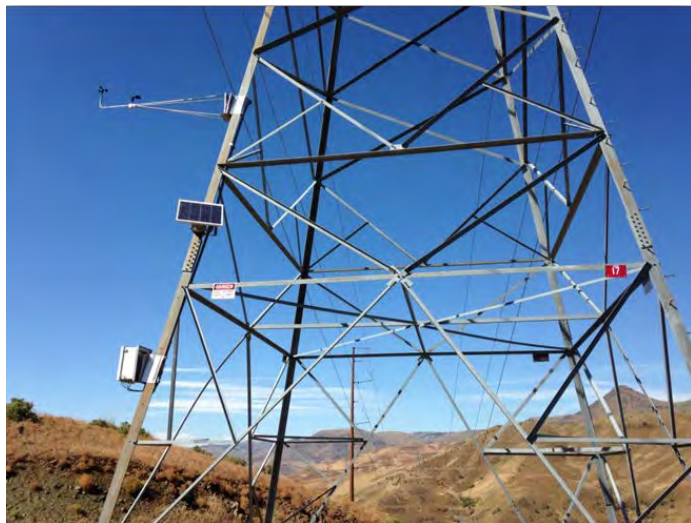
Figure 2. Dynamic line capacity equipment installed in Hells Canyon
