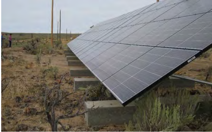
Figure 1 Solar installation as part of the Solar End-of-Feeder Project
