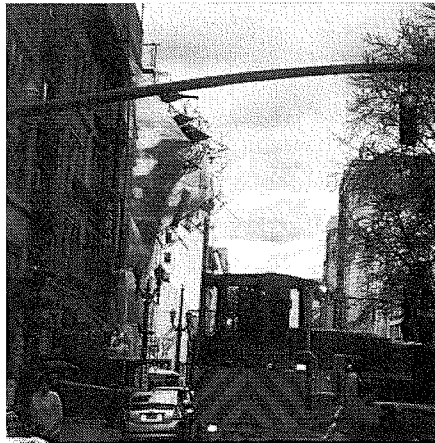
Scaffolding on a building project located at Southwest Fourth and Washington came crashing down on the street, hitting at least one vehicle. Photo by Byron Beck
