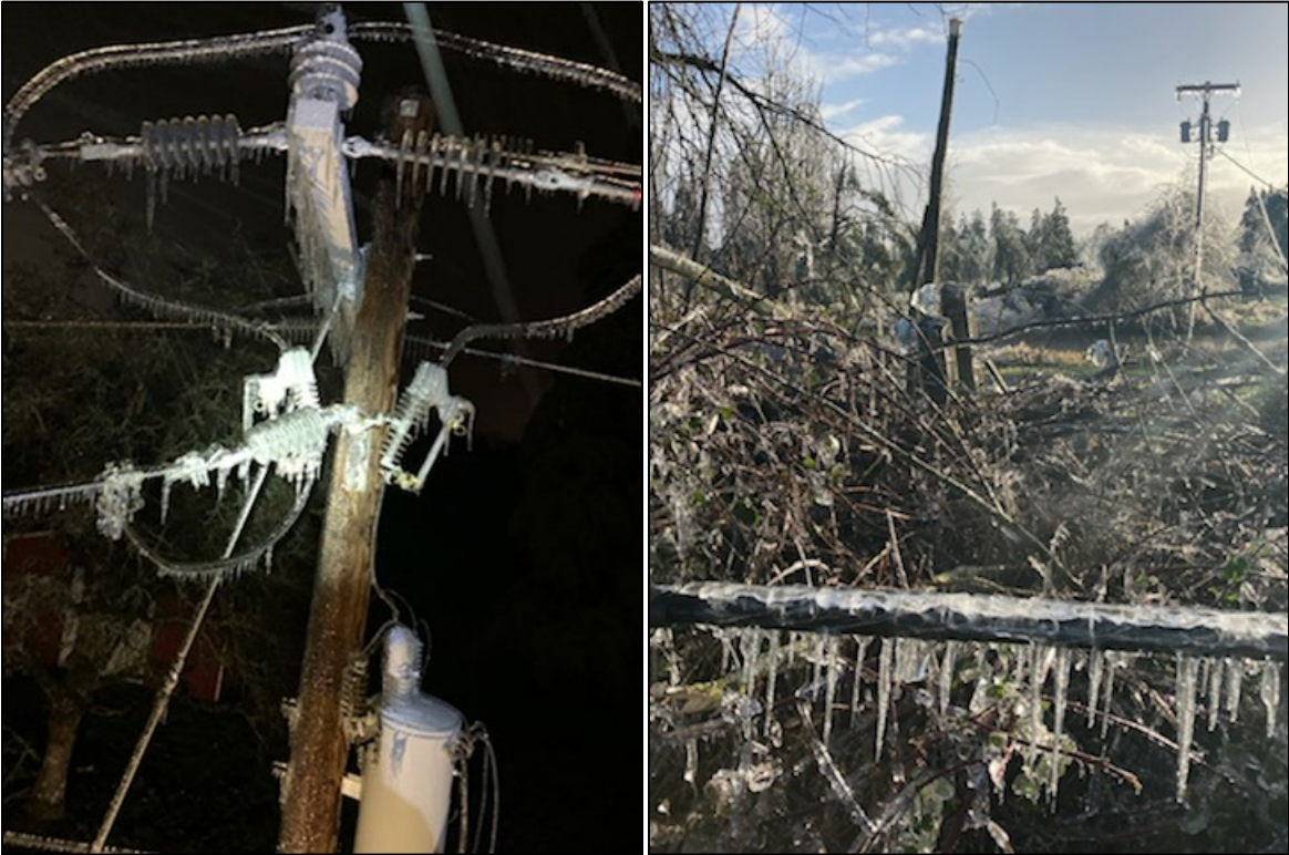
Figure 7: Storm photos and the effects on system facilities.
