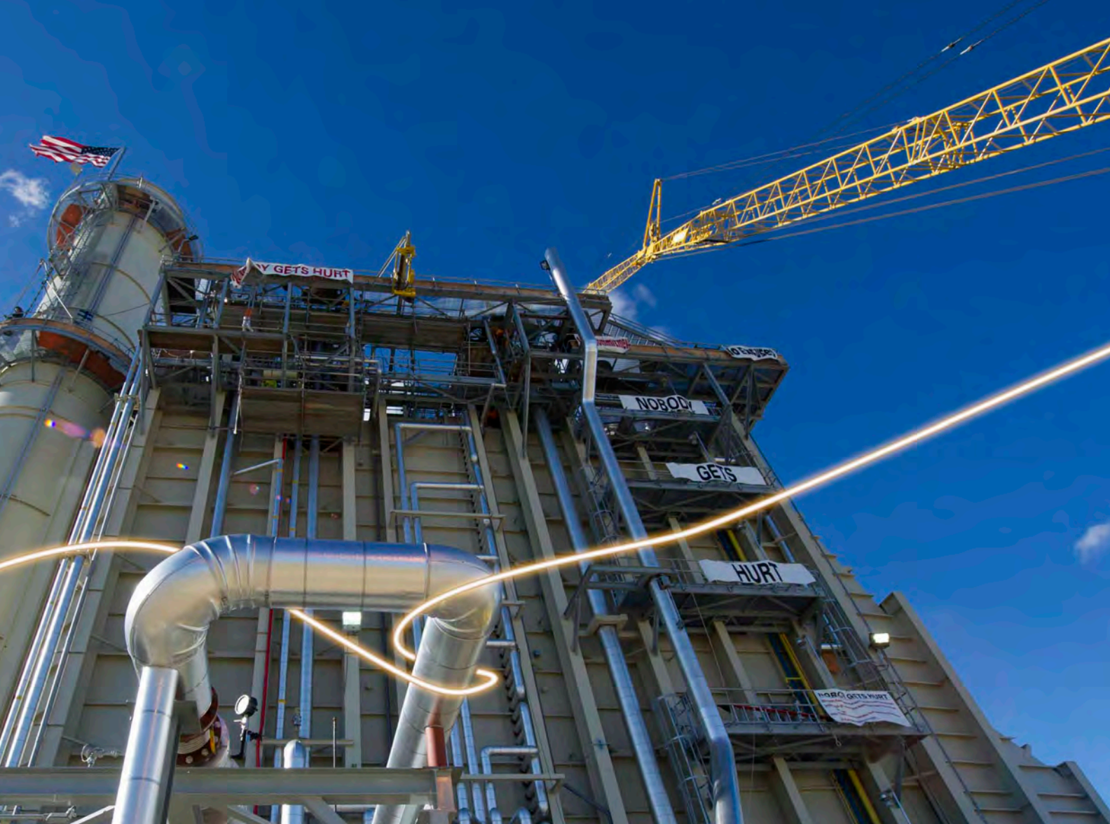
Langley Gulch Power Plant
