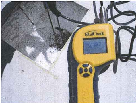
Testing of facer where moisture was observed on polyiso insulation.
