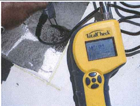
Moisture reading taken at surface of vapor barrier at joint of insulation.
