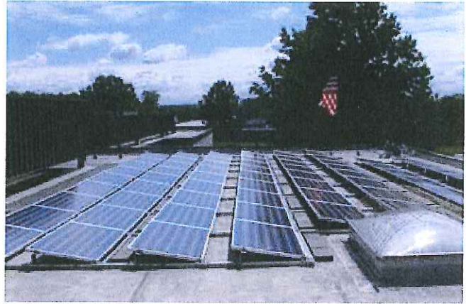
Open air design for increased energy production.
