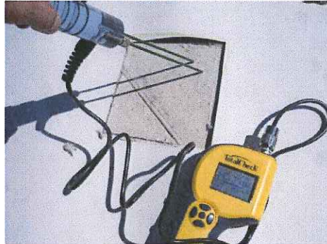
Moisture readings taken at facer of cover board.
