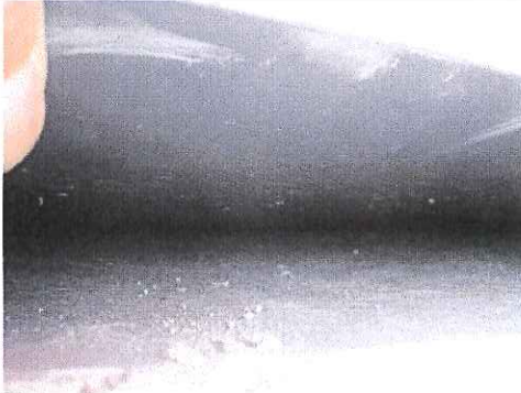
View of underside of membrane where moisture was observed.
